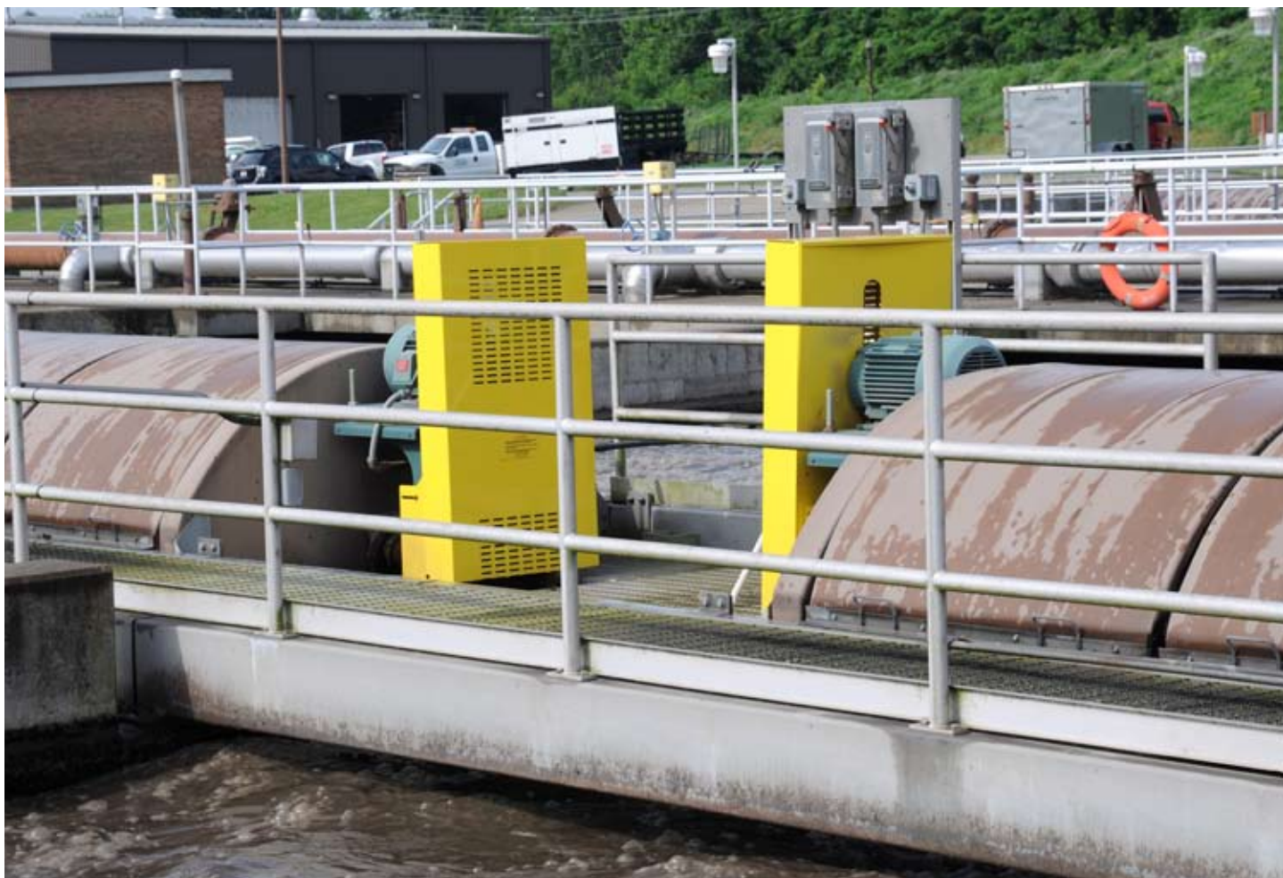
When equipment needed to be replaced on the existing Vertical Loop Reactors (VLRs) at the Lower Little Miami Wastewater Treatment Plant, Warren County officials chose Baldor equipment. VLRs are an aerobic biological treatment process that utilizes large discs that are continually rotated to move wastewater and impart oxygen for aeration.
